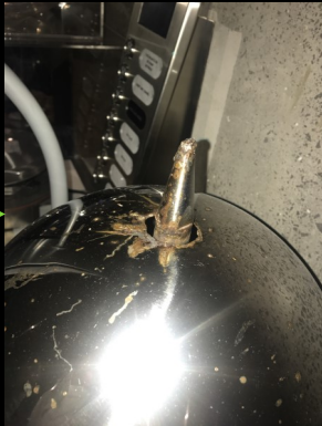
ERICO DYNASPHERE AFTER BEING AFFECTED BY LIGHTNING STRIKES
