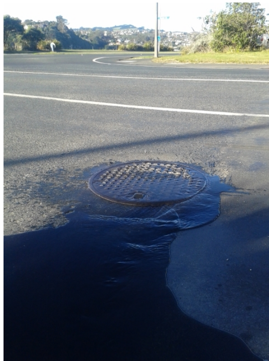
Figure 39. Sea water rising up through the stormwater system on Teviot Street at about high tide, 2:30pm on 6 May 2016. The pressure in the stormwater pipe below this man-hole cover is such that it has pushed water up above ground level. This was not the highest tide experienced during that month. Photograph source, ORC.
