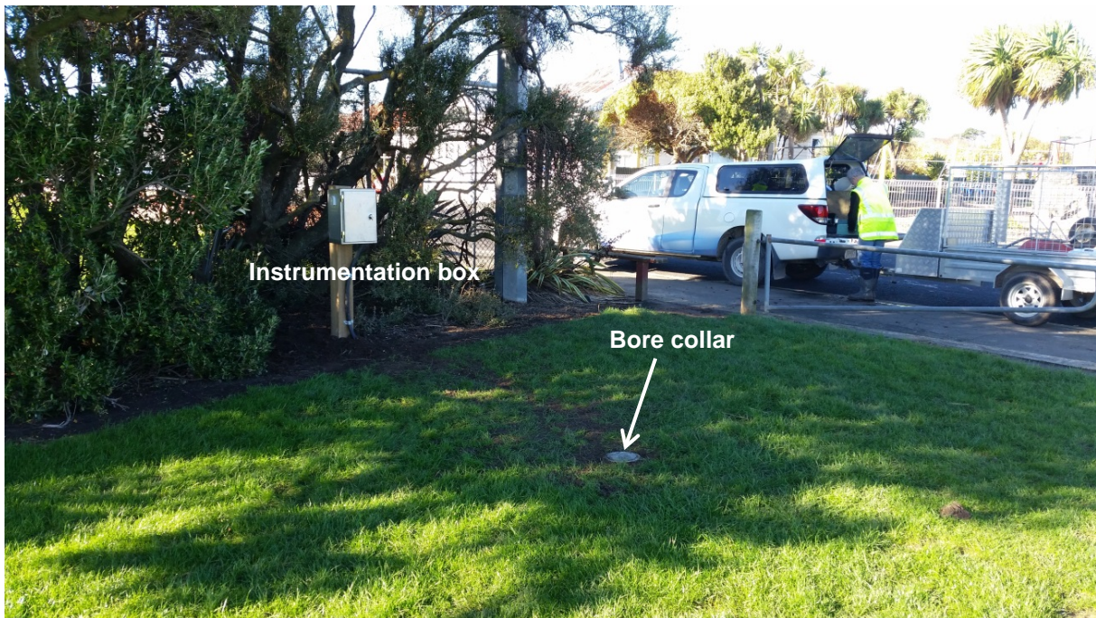
Figure 17. Typical example of an ORC bore installation, with bore collar and instrumentation box, at the Culling Park site.
